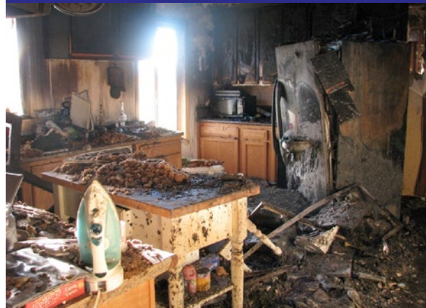
Figures 121, 122 and 123. February 2017 Beaumont, California Explosion of Extraction Lab, Marijuana Concentrates, and Butane Canisters.
